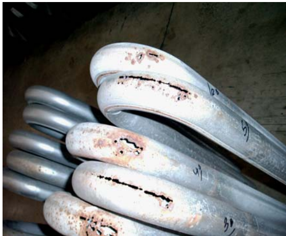
Figure 2: Corroded Aluminized Steel Heat Exchanger
